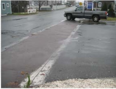
Faded crosswalk at the southern end of Shank Painter Road, looking westbound along Bradford Street.
