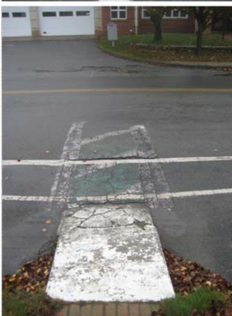
Faded crosswalk between the Police Station and Fire Station.
